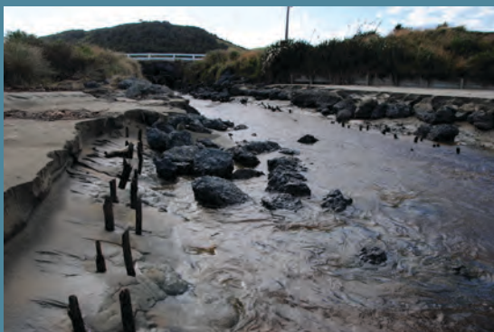
Erosion at the mouth of Cook Creek - 9 February 2011
